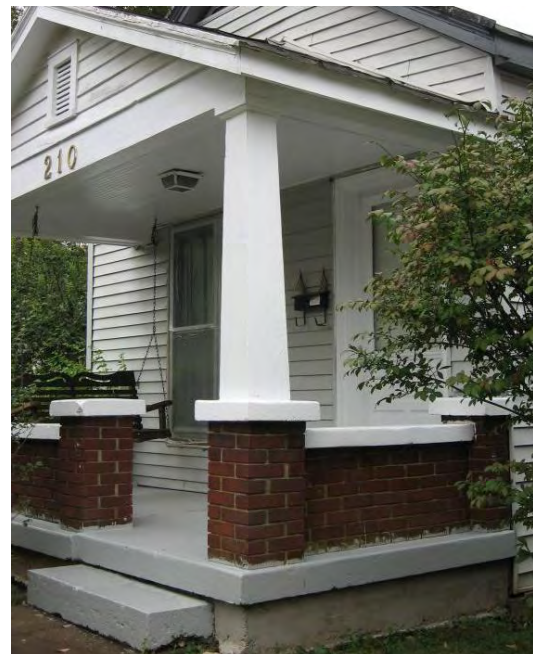
Craftsman posts like those at 210 East John Fitch Avenue can be ordered from milling companies.
