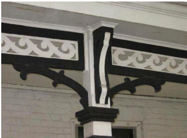
Wood, like that used for the trim at 227 North Third Street, is a traditional material for porch elements.
