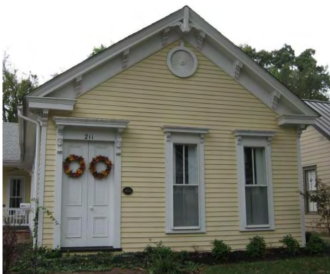
Brackets, gable returns, and window and door cornices all help define the mid 19th century Italianate style of the house at 211 East Flaget Avenue and must be retained to protect its integrity.
