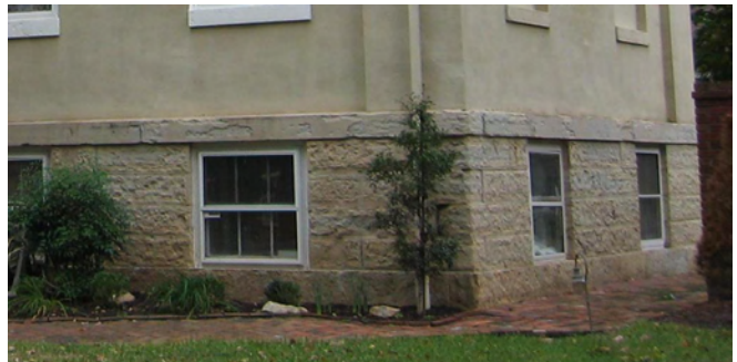
Repairs made to the stone foundation at 402 North Third Street should be in keeping with the masonry guidelines.
