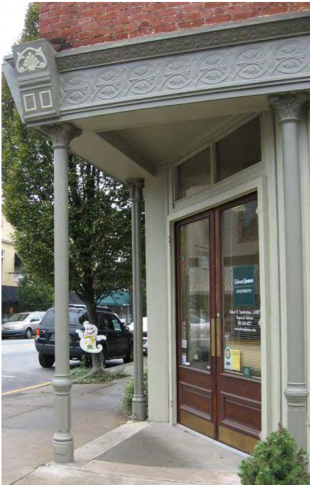
Maintain the painted surface of features like the cast iron columns and pilasters at 130 North Third Street.
