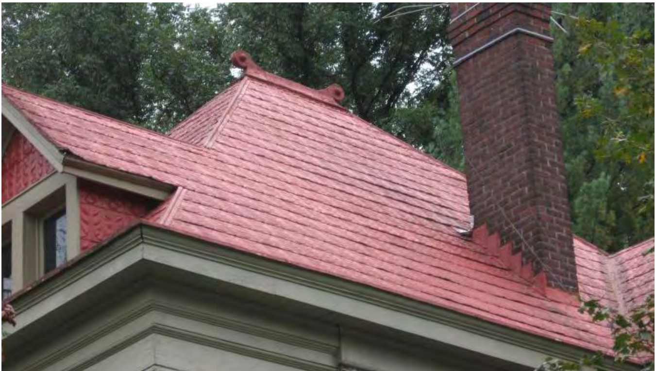
Cresting and pressed-metal shingles add to the historic character of the house at 117 West Broadway Avenue.
