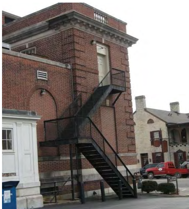
The fire escape on the Nelson County Public Library building on Public Square appropriately used placement behind and close to the building.
