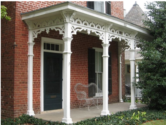
If deterioration occurs on historic porches such as the one on 206 South Third Street, deteriorated areas should be removed and replaced.
