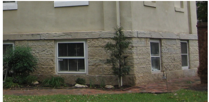
Repairs made to the stone foundation at 402 North Third Street should be in keeping with the masonry guidelines.
